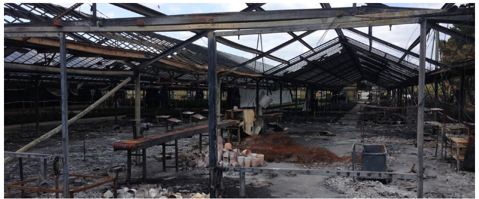
Fire damage at Oasis Horticulture.
