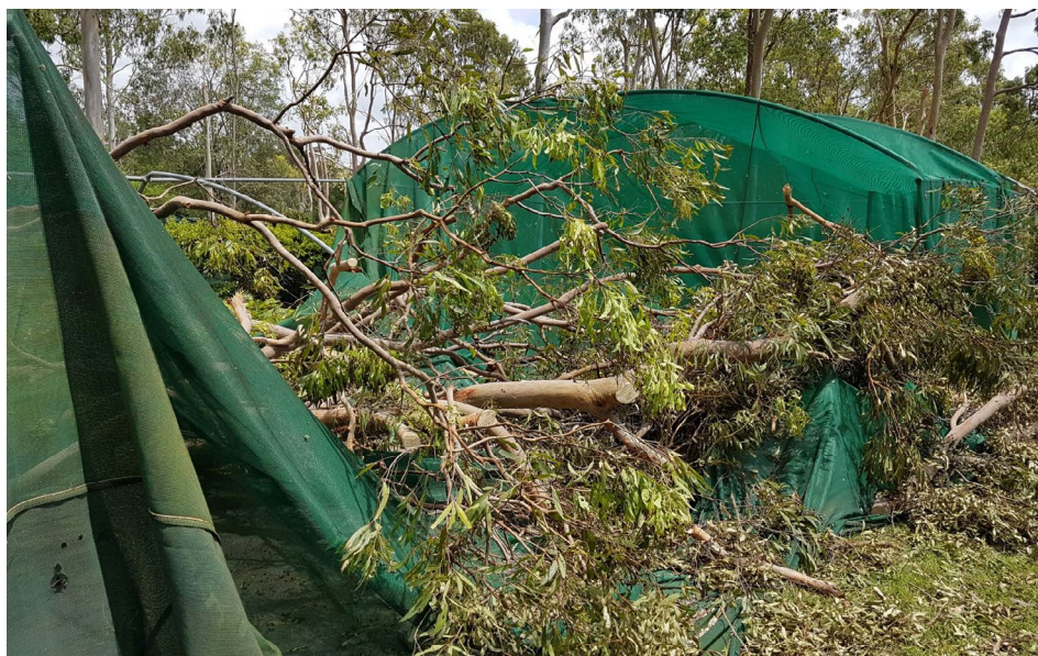
Fallen tree on a shadehouse.
